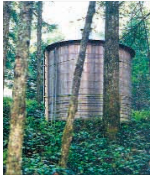
Goldstream Park Provincial Park (right). This illustration shows how even a large utility structure, if a simple, single form, is unobtrusive. The cylindrical wooden water tower with a galvanized steel conical roof provides a corner-less form within the forest landscape.
